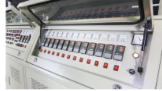
Operation Control System
